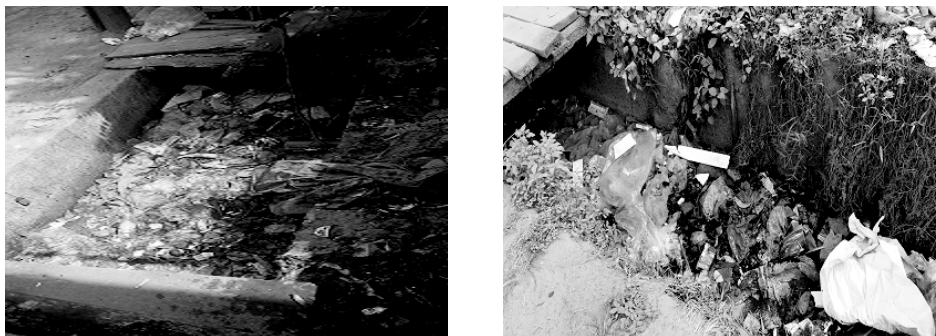
Figure 4: Two specimen pictures of blockage in sewerage system in Feni town.
