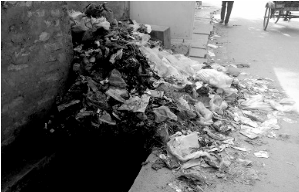
Figure 5: The obstruction in the sewerage system created by the daily wastage in Feni town.
